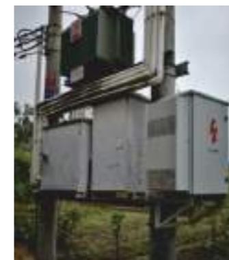
Southern Power Grid Cooling
