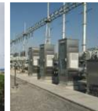
State Grid Cabinet Cooling
